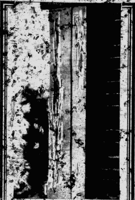
Due to lack of protection, the destructive power of White Ants was so certain in this structure as to render it useless in an incredibly short time.
