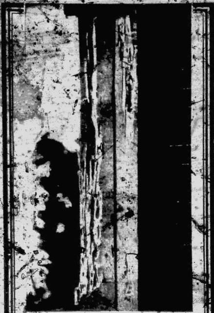
Owing to lack of protection, the destruction caused by White Ants was so great that this structure as to render it useless in an incredibly short time
