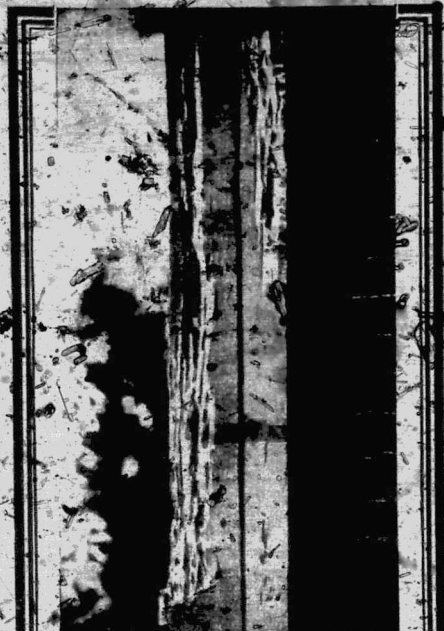
Owing to lack of protection, the destruction caused by White Ants was great in this structure. It is rendered useless in an incredibly short time.
