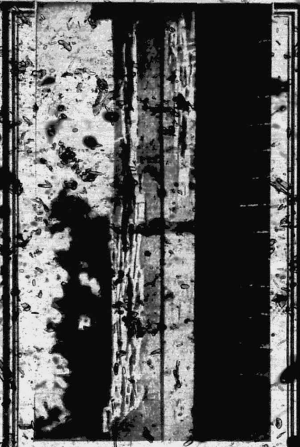
Due to lack of protection, the destruction caused by White Ants was great in this structure as evidenced by the mass insect damage shown here.
