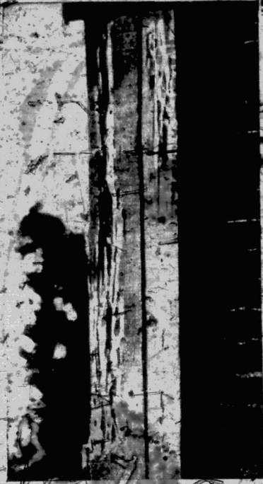
Due to lack of protection, the destruction caused by White Ants was so great the structure as to render it useless in an impossibly short time.
