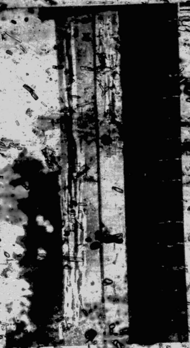
On the left, a picture of a structure destroyed by White Ants. On the right, a picture of the same structure as to render it useless and irreparably damaged.
