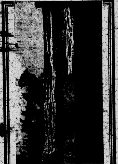
Owing to lack of protection, the destruction caused by White Ants was so great in this structure as to render it useless in an incredibly short time.
