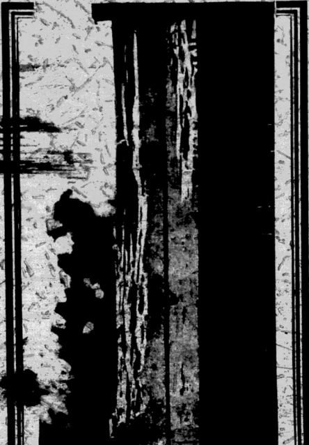
Due to lack of protection, the destruction caused by White Ants was so great in this structure as to render it useless in an incredibly short time.
