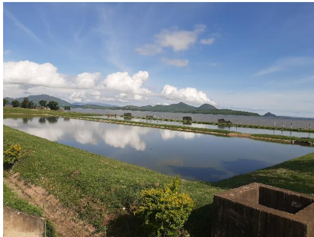
Figure 10: Homa Bay Sewer Treatment Plant.
