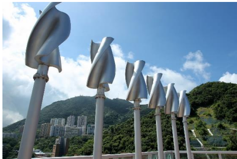
Figure 49 Image showing vertical-axis of installed wind turbines on top of a building at the Hong Kong University campus.
