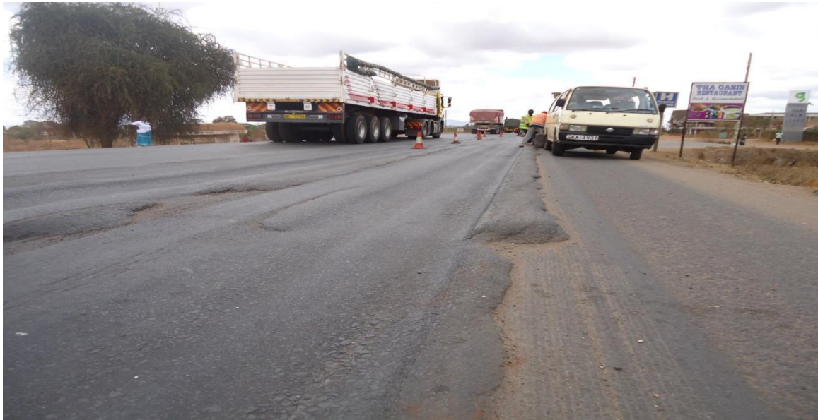
Figure 1.5: Rutting on Mombasa Road, Makindu Town
