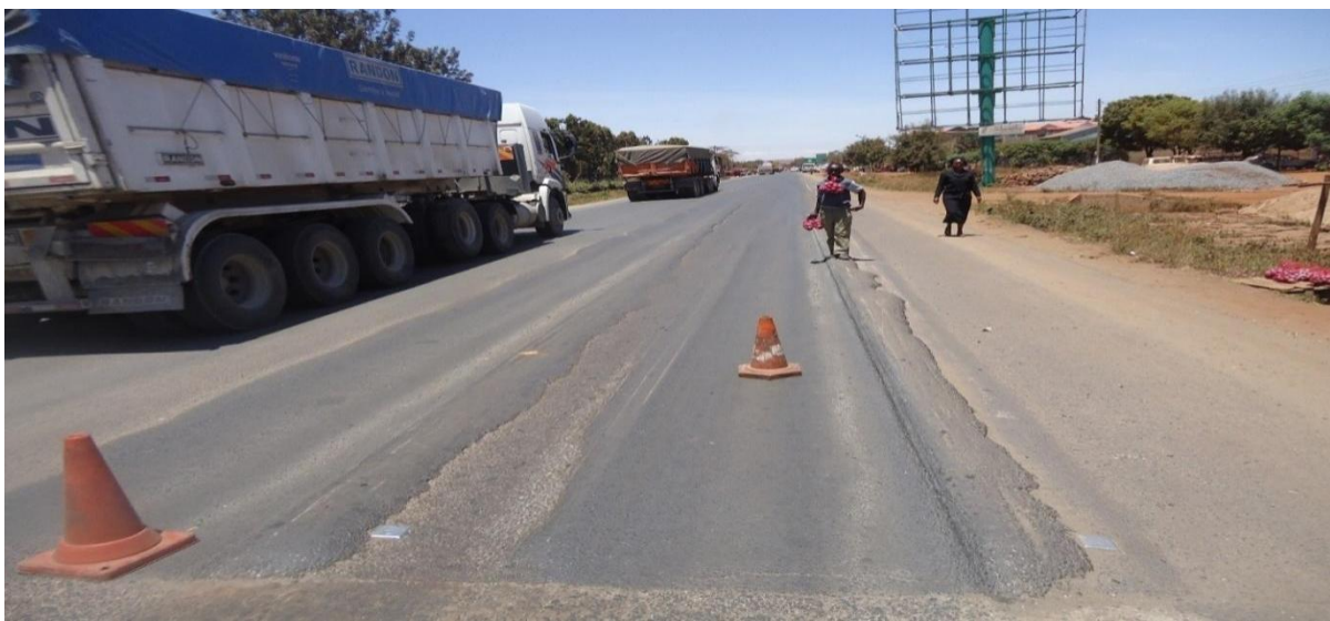
Figure 1.1: Rutting on Mombasa Road, Machakos Turn off
