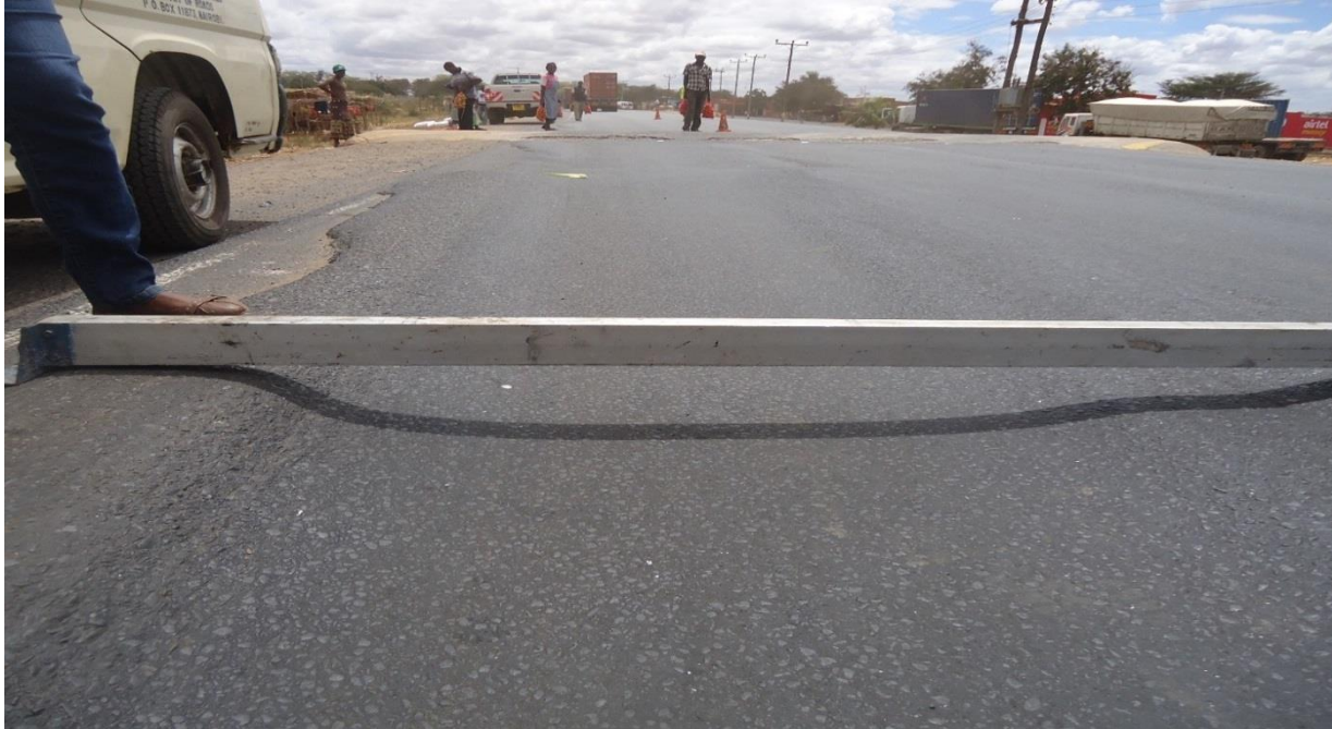
Figure 1.4: Rutting on Mombasa Road, Emali Town
