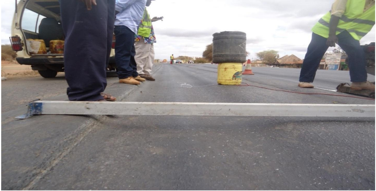
Figure 1.2: Rutting on Mombasa Road, Salama Town
