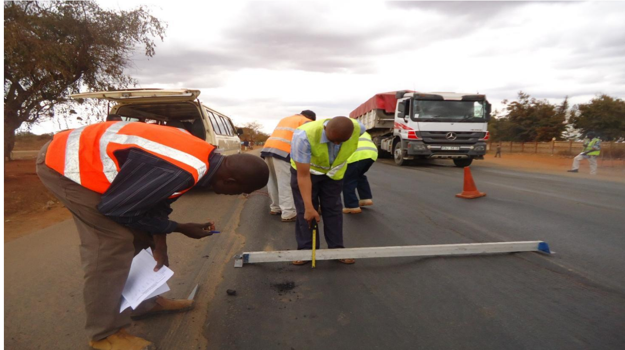
Figure 1.3: Rutting on Mombasa Road, Sultan Hamud Town
