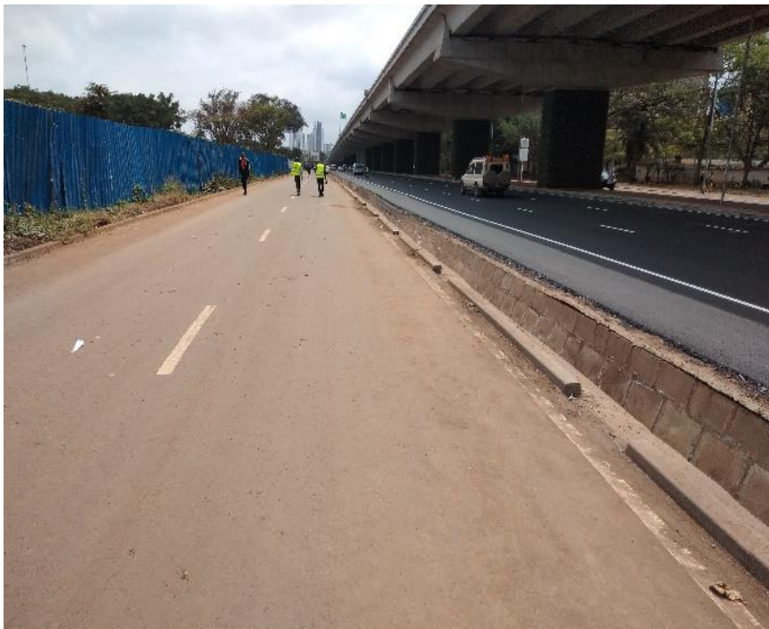
Plate 3-4: Open Drains along Uhuru Highway, Source: Author, (2022)
