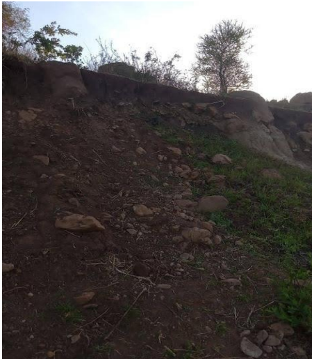
Gully erosion at the bank of River Tana
