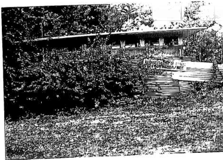
Plate 10;- The rear view of On-going rehabilitation works at the toilet block along Nyerere road- an NCBDA –CCN joint project.
