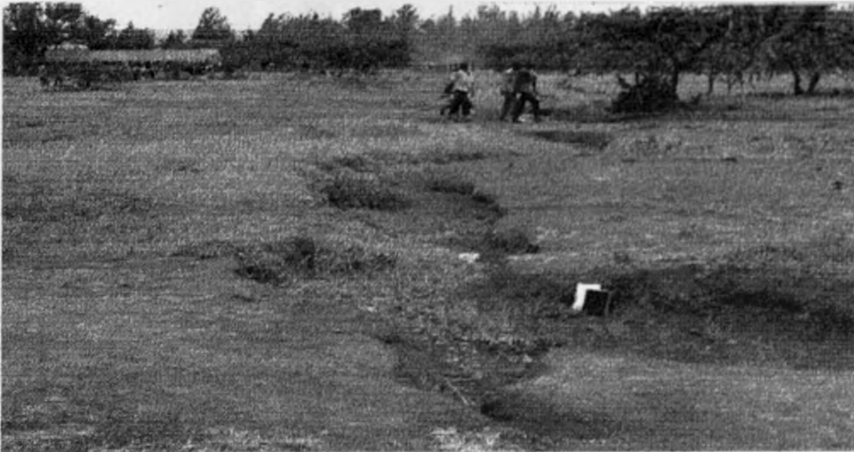
PLATE 6.6 A gully in the making inside the market grounds. Such are accelerated by the effect of heavy vehicles on the bare ground. (Please notice the notebook indicating the depth)
