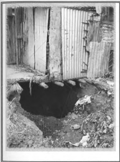
Photo 4.5: Direct drainage of latrine effluent into river/open drain (Source: Fieldwork)
