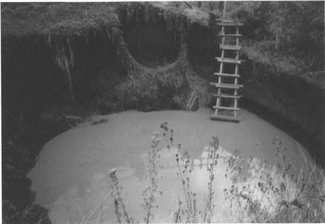
Plate 4.4: Water pan with collapsed walls
