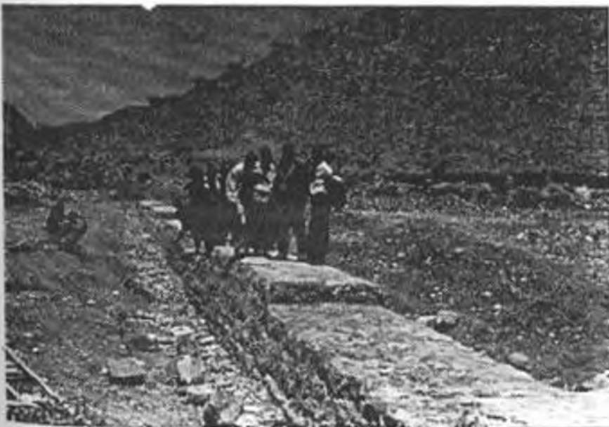
Plate 4.4 Diversion structure built across Shugala river by DHP (photo by Dr. Nashon K.R. Musimba, 1997)
