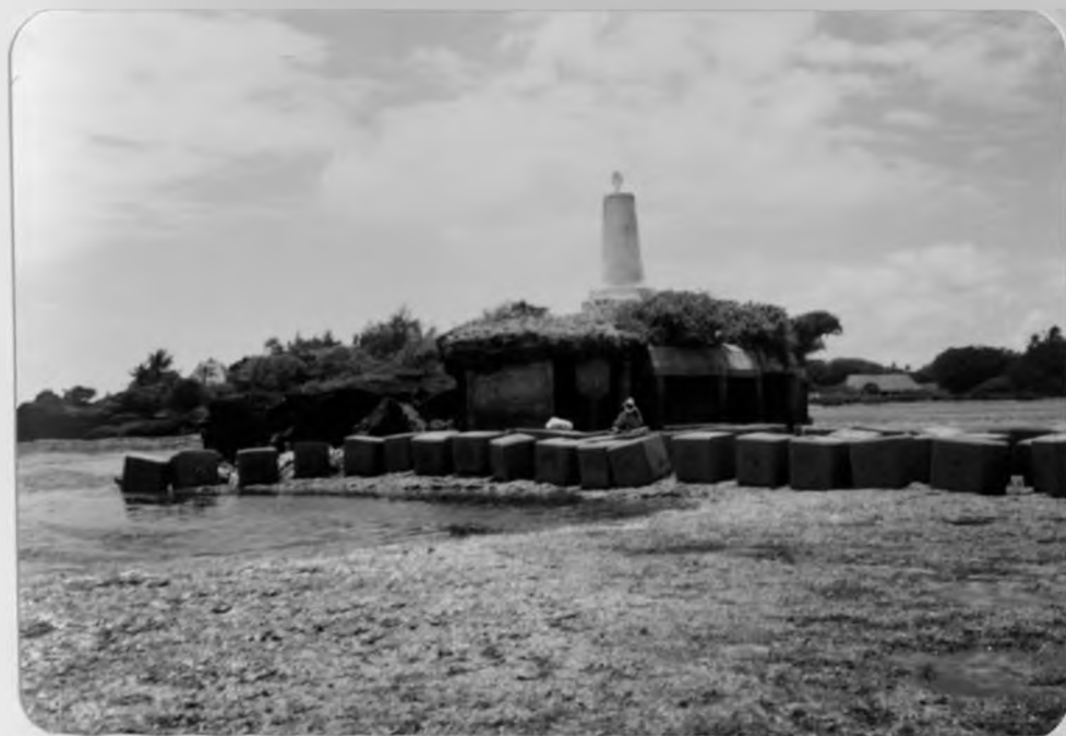
Plate 4. Concrete slabs placed in front of the monumental Vasco da Gama Pillar for protection against wave erosion.
