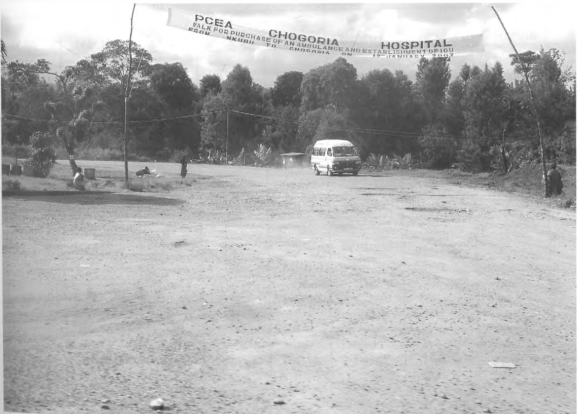
New Road Condition. Evidence of potholes and tarmac surface basically worn off due to lack of maintenance. (Photo by Author: April 2007)
