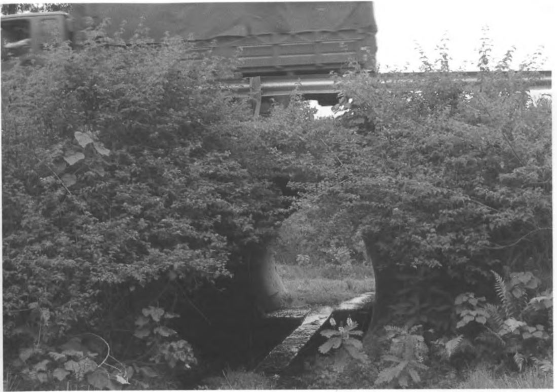
Plate 8: Culvert improvised to serve as a tunnel for domestic animals and small farm tractors at Kaguru Farmers Training Institute (Photo by Author, 2007)
