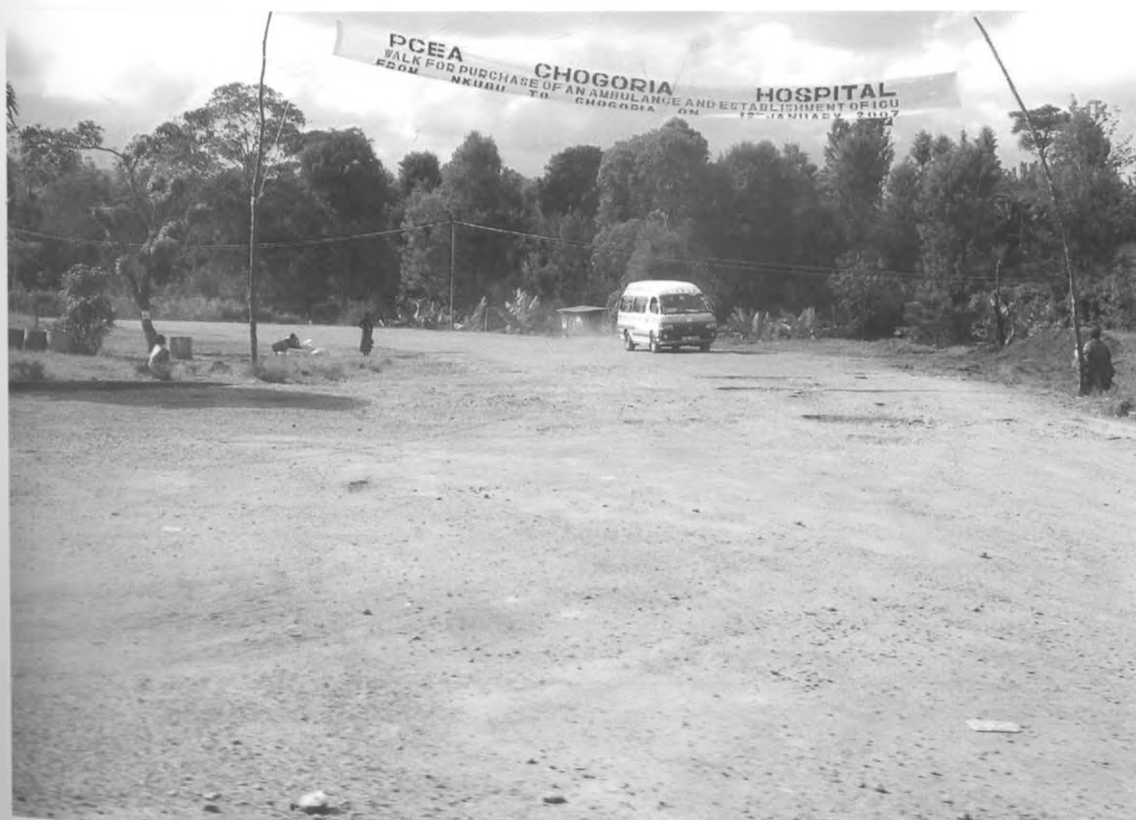
New Road Condition. Evidence of potholes and tarmac surface basically worn off due to lack of maintenance. (Photo by Author: April 2007)
