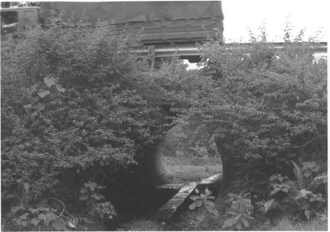
Plate 8: Culvert improvised to serve as a tunnel for domestic animals and small farm tractors at Kaguru Farmers Training Institute (Photo by Author, 2007)
