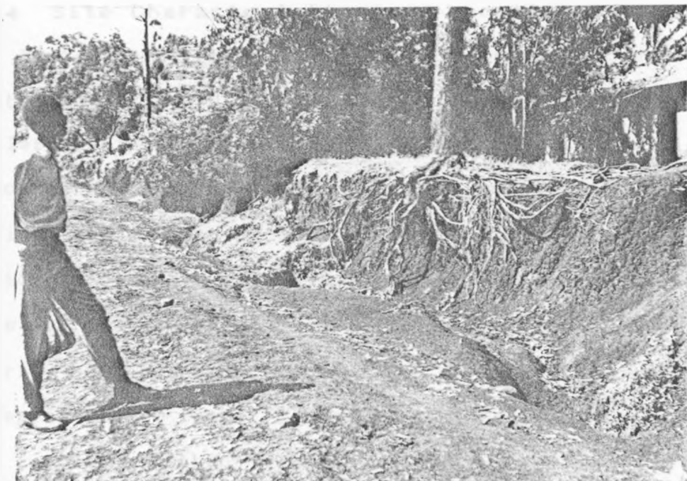
Plate 5.2: The stormwater has eroded the Daraja Mbili- Nubia road. Notice the exposed roots of the tree indicating massive soil erosion. The sides of the road form the channel for stormwater drainage.
