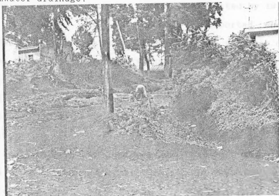
Plate 5.3: Stormwater carry a lot of sediments. The small size of the culverts constrain water passage. As a result they are blocked.
