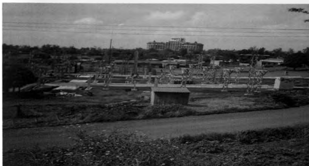
Plate 4-4 Ruiru Power Sub Station
