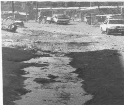
Plate 3.4 Sewerage Run-off on road.
