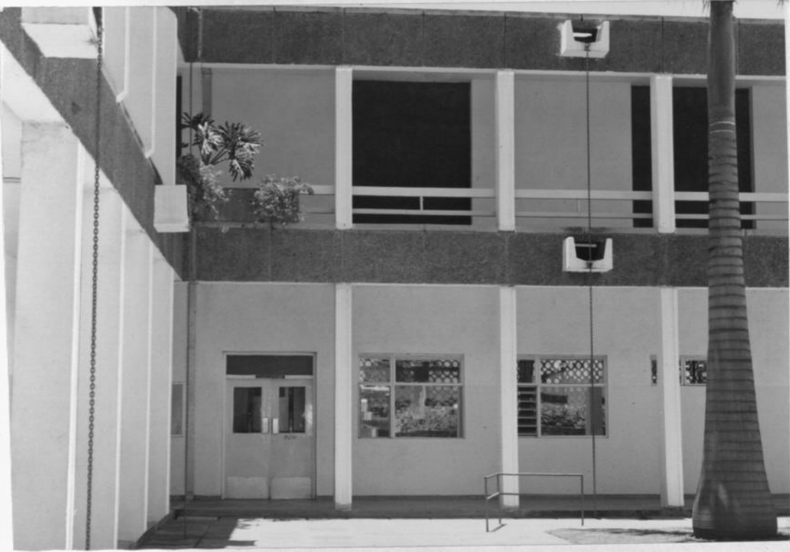
PLATE IV A CHAIN ACTING AS THE DOWNPIPE TO A FLAT ROOF
