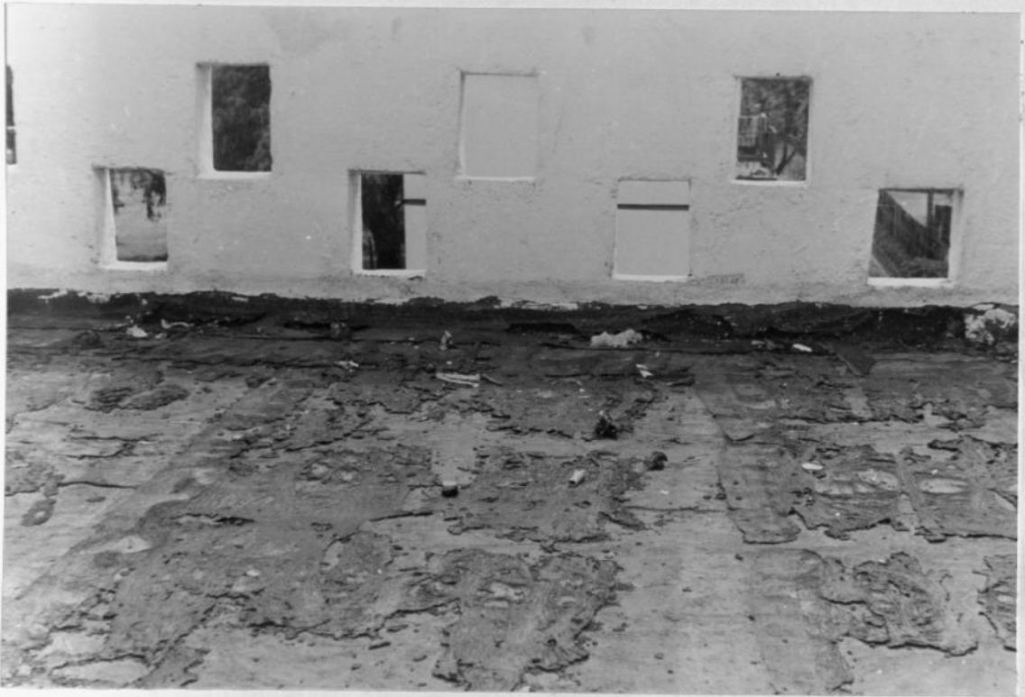
PLATE II BUILT-UP FELT ROOF SHOWING THE EFFECTS OF EXPOSURE DUE TO LACK OF REFLECTIVE FINISH
