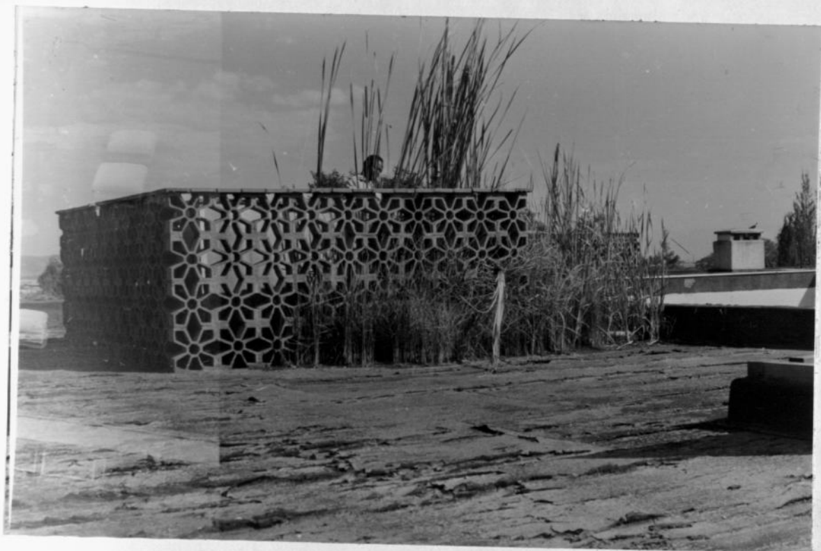
PLATE III WILD PLANTS GROWING AROUND A BLOCKED OUTLET LONG FORGOTTEN BY THE MAINTENANCE TEAMS
