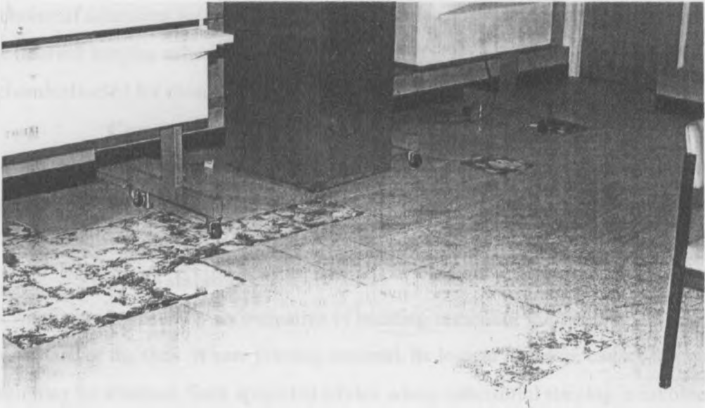
Photo 2 Lifting plastics tiles over defective damp proof membranes (see also 7.2.13)
