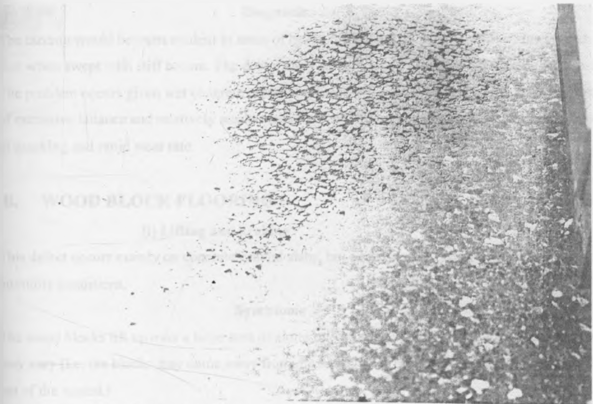
Photo 1 Breakdown of terrazzo finish at a buffet checkout caused by a combination of wear and spills of milk and other food stuffs.
