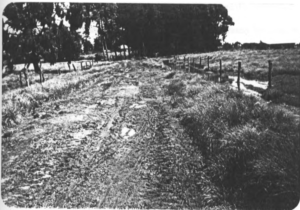
Plate 11: Poor State of the Roads Necessitate the Use of NMTs.
