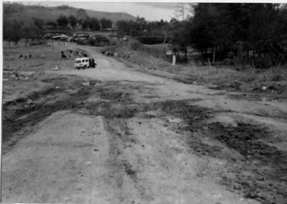
Plate 4-8: Potholes on a Road in Kipkelion
