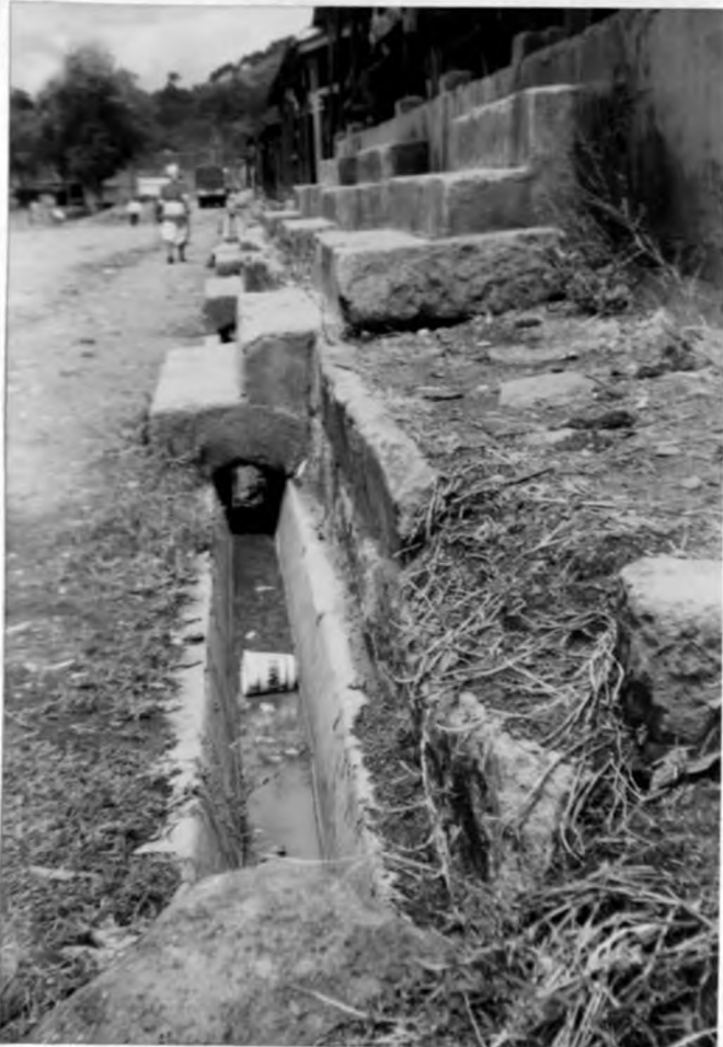
Plate 4-6: Sullage on Open Drains
