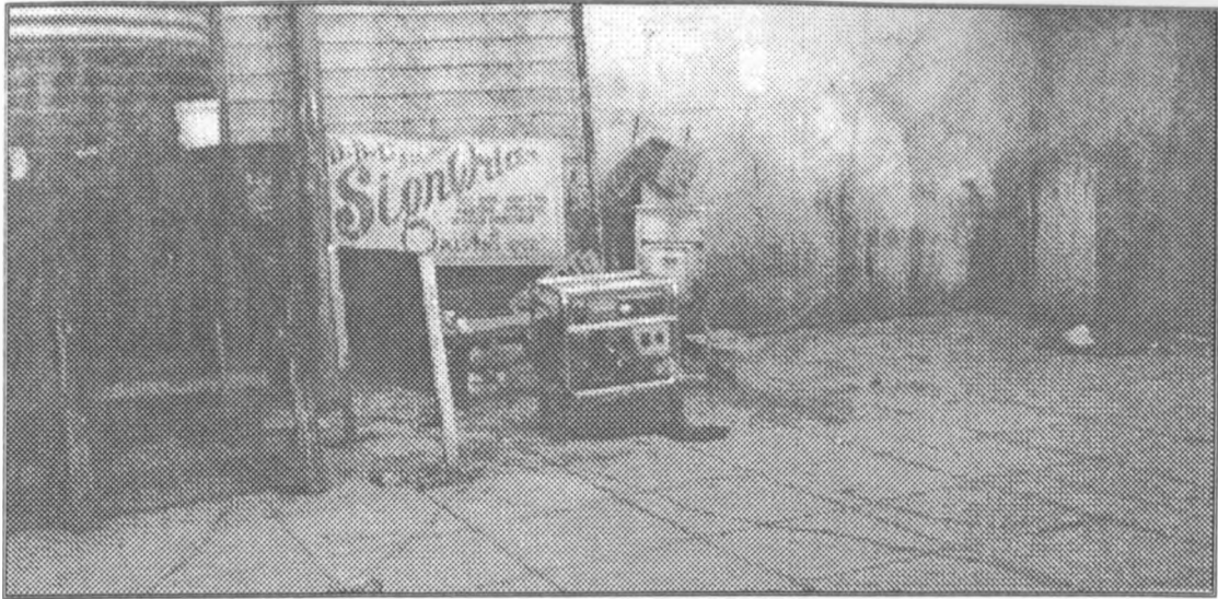
Plate 5-11 The Generator In Kenyatta Market
