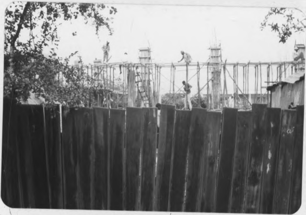
PLATE 3: Workers in precarious work positions. This signifies the attitude of workers and management towards site safety.
