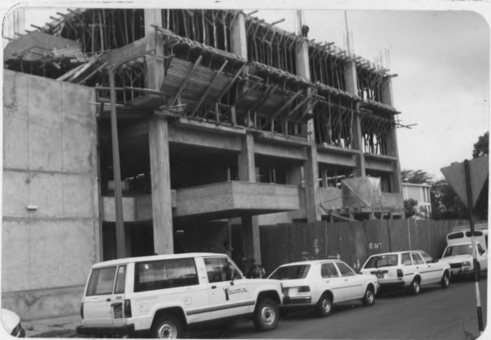
PLATE 4: Inadequate protective hoarding on a site where part of the building under construction is already in use. This poses grave danger to the users.
