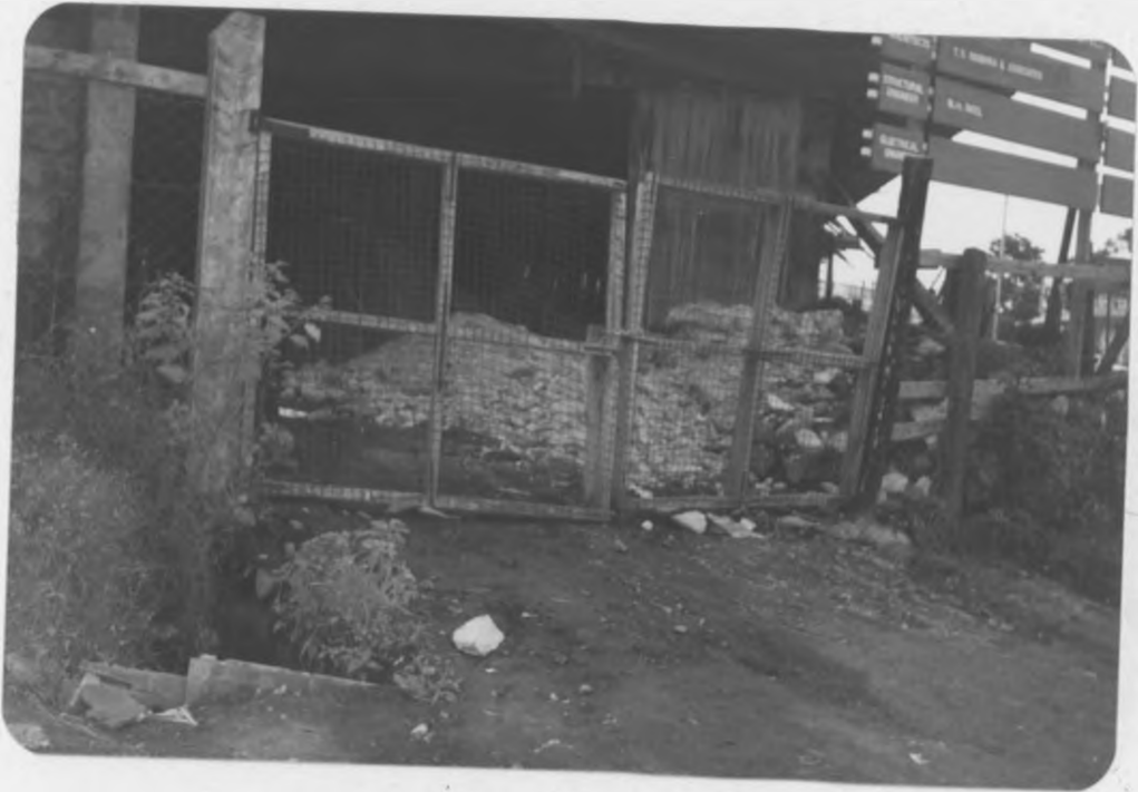
PLATE 1: An obstructed site access. Note the debris laying just inside causing obstruction to the already restricted access.
