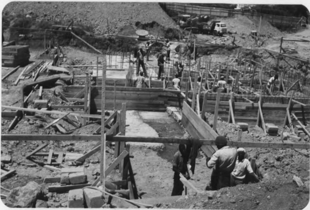
PLATE 2: A relatively clean and unrestricted site. Note workers without proper protective gear.
