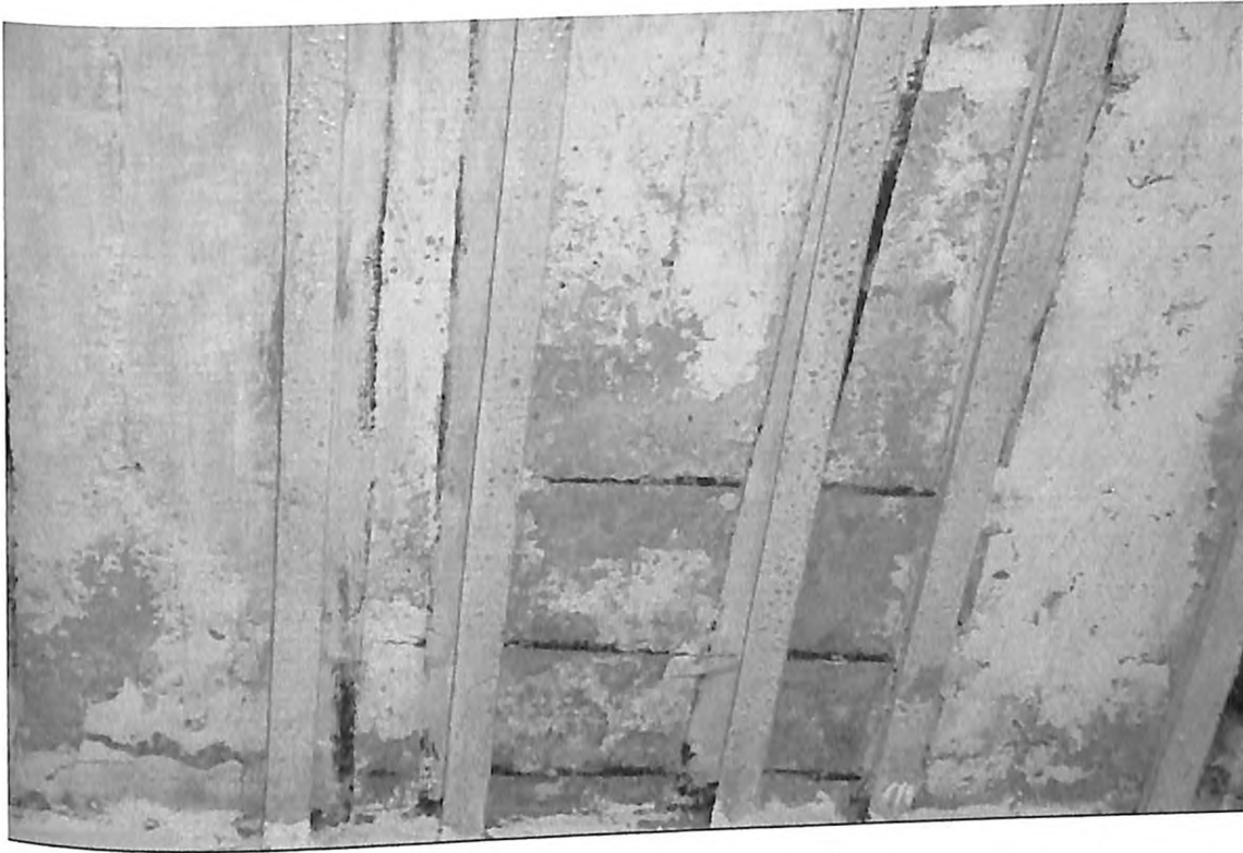
Plate 5.3 A flaking wall showing cracks and traces of salts.
