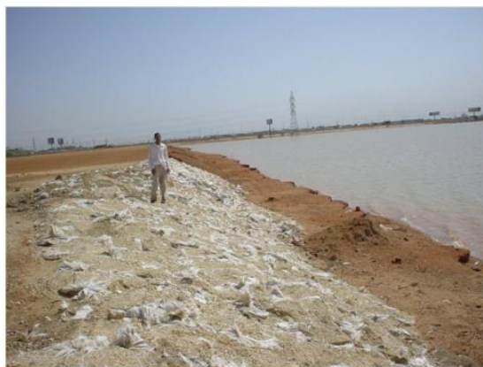
Figure 5-7: White Nile eroded bank
