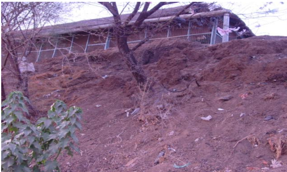
Figure 4- 13: River bank erosion at Forestry Department Rest House at AlSuki
