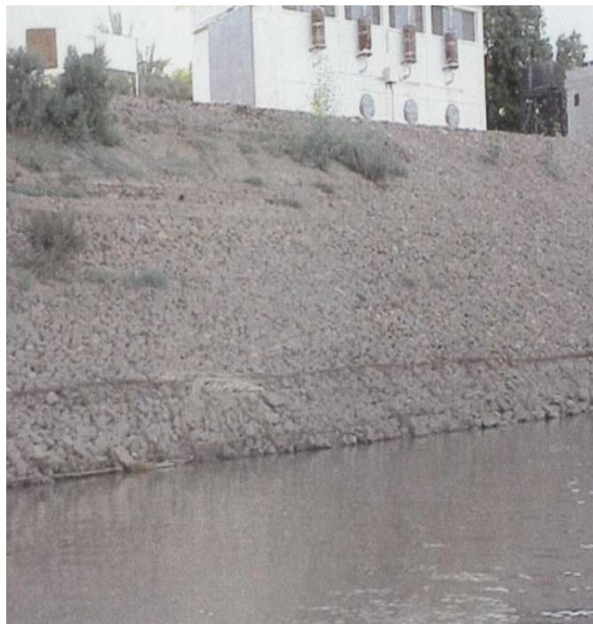
Figure 3- 8: Protection of pumping station at El-Gaba –Northern State by rock and cement
