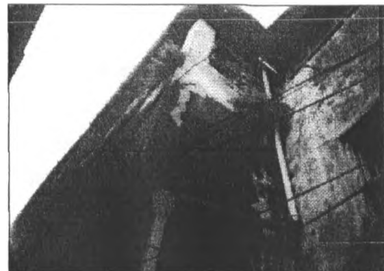
Unsightly Down Pipes With Vegetation
