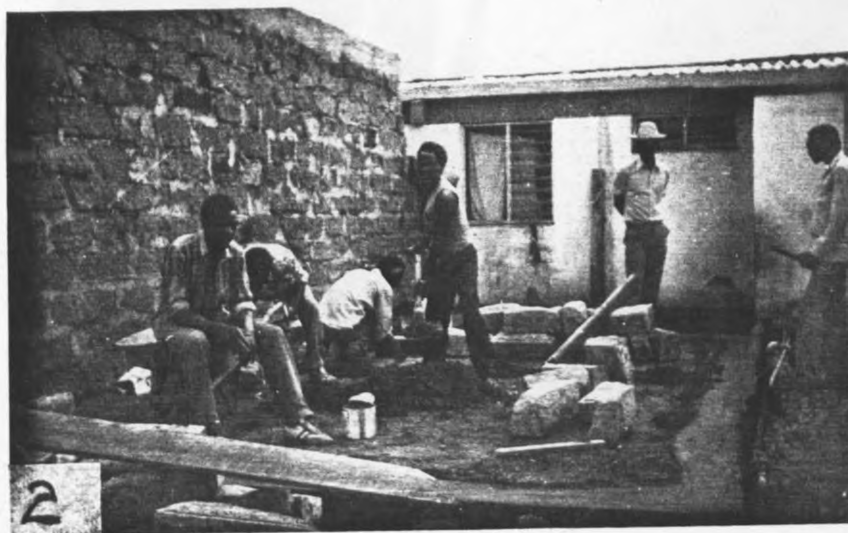
PLATE 2: Completing a slab for a front extension. Note : The wall of a neighbouring extension.
