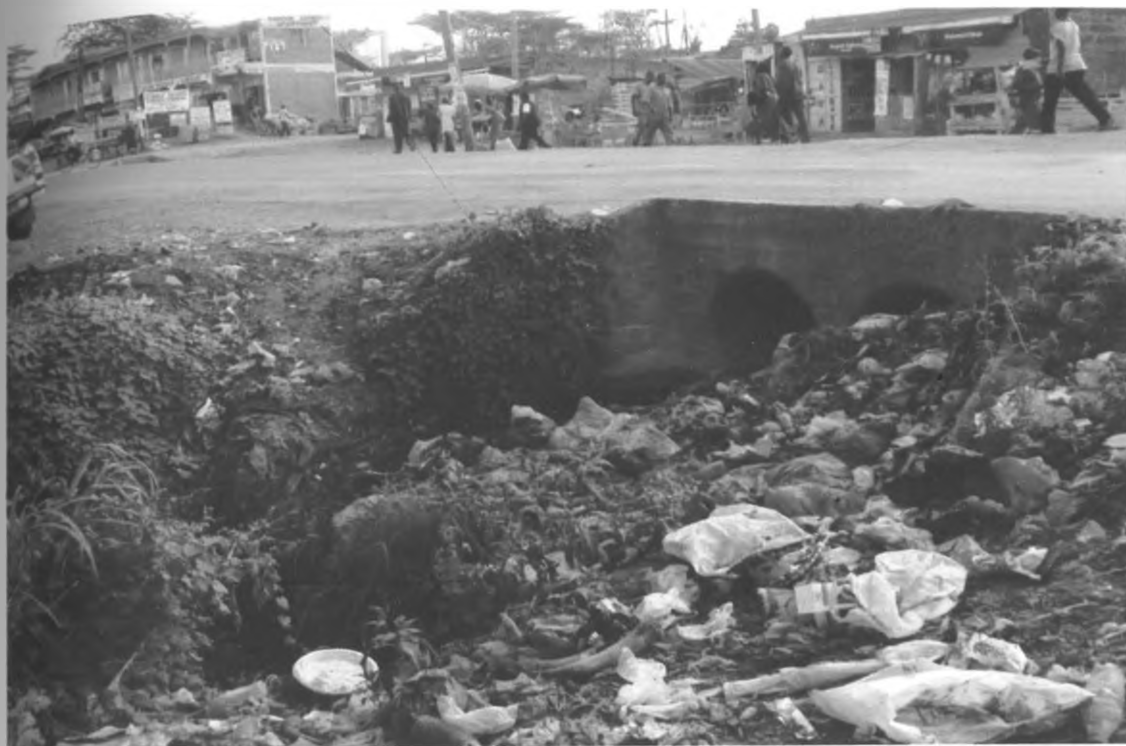
Photo 6.3: Solid Waste Dumped on Drainage within the Town
