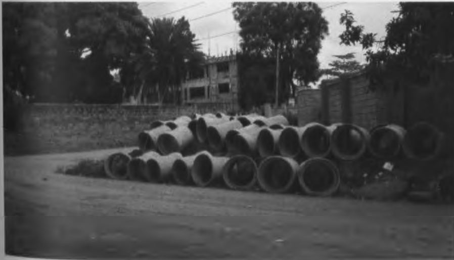
Plate 5.13: The expansion of Sewerage System along Okoth Aura Road in Section A
