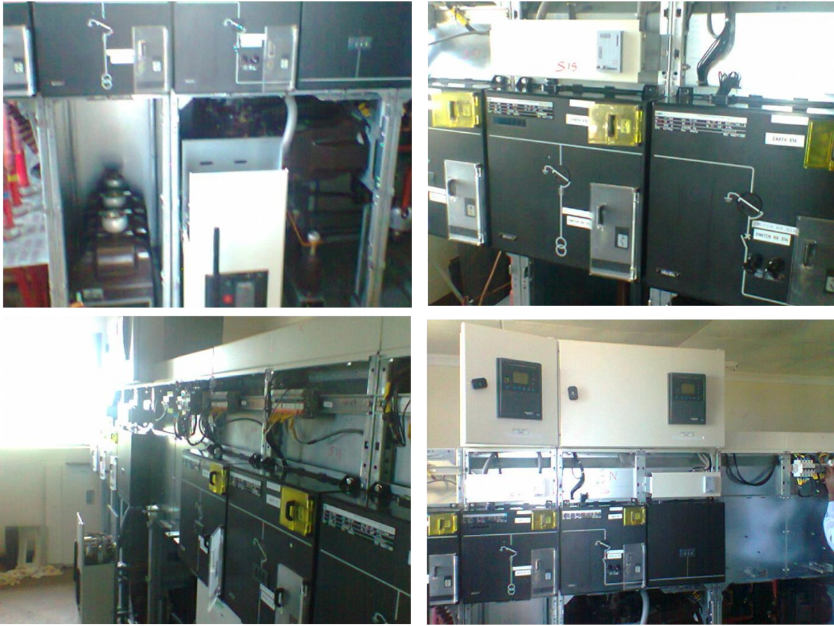
Figure 3.2 Control and switching centre at the Ngong Wind Farm
