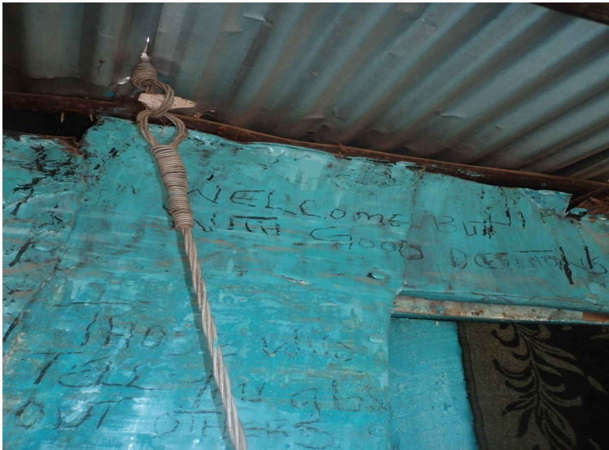
Figure 15: Pole Support inside a House
