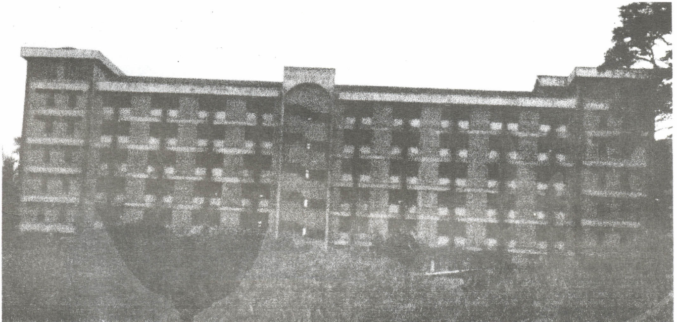
An incomplete hostel at the lower Kabete campus that can accommodate over 1000 students.
