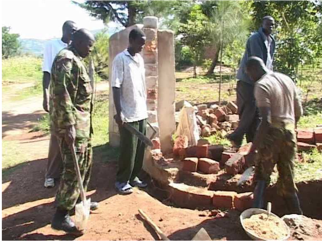
Fig.7: KDF Army Engineers and local civilian volunteers rebuilding damaged buildings in Mt. Elgon Conflict areas.
