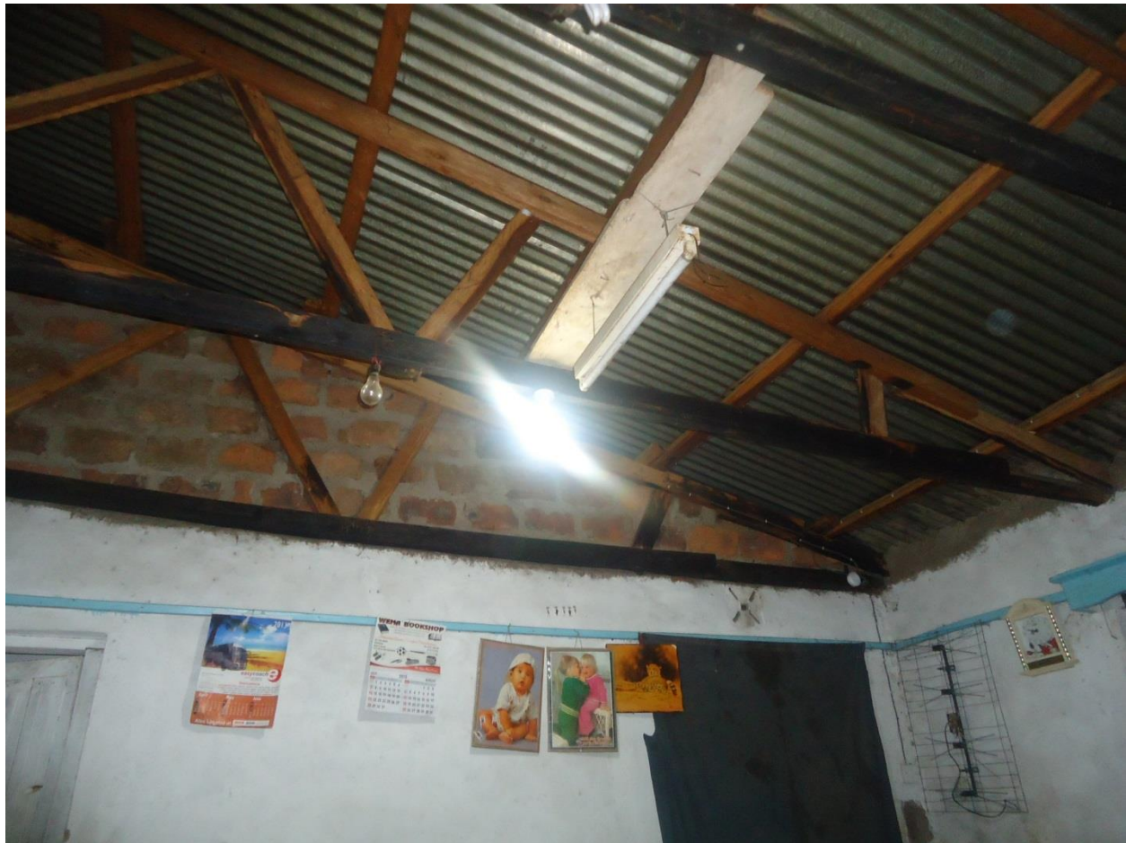
Figure 4.7: PV Solar power used for Lighting in Borabu Household
