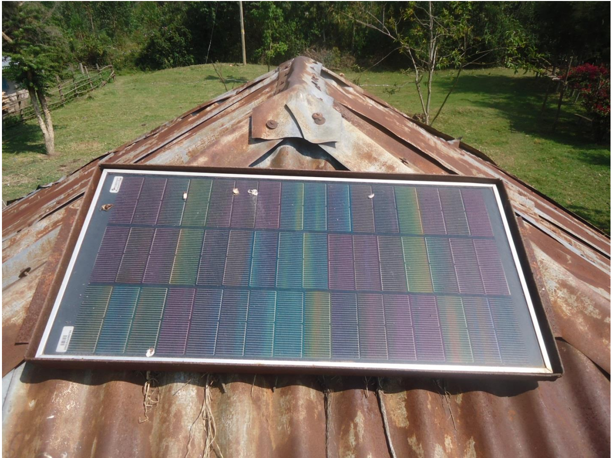
Figure 4.5: PV Solar System on the Roof.
