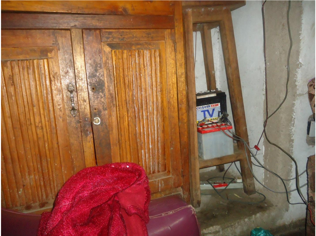
PV solar system power transmitted into the battery directly without passing through the inverter.
