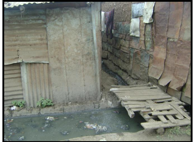
Plate 1.10b: Poor drainage channels in Huruma
