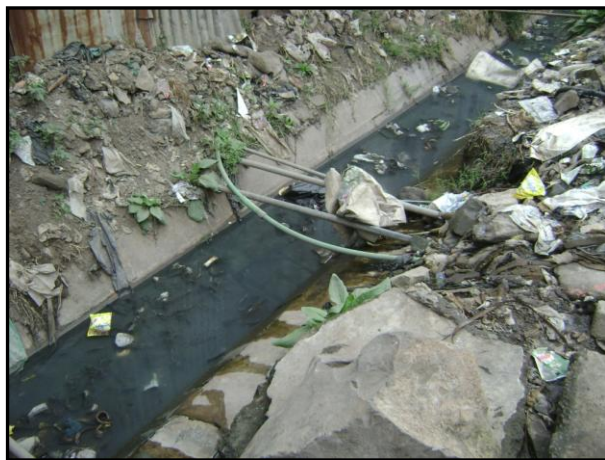
Plate 4.17a: Illegal water connections in Huruma, Nairobi
