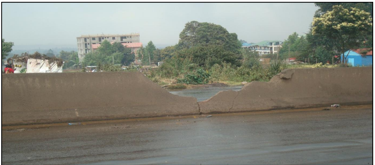
Picture 8: Broken barriers which can be used for grade crossing
