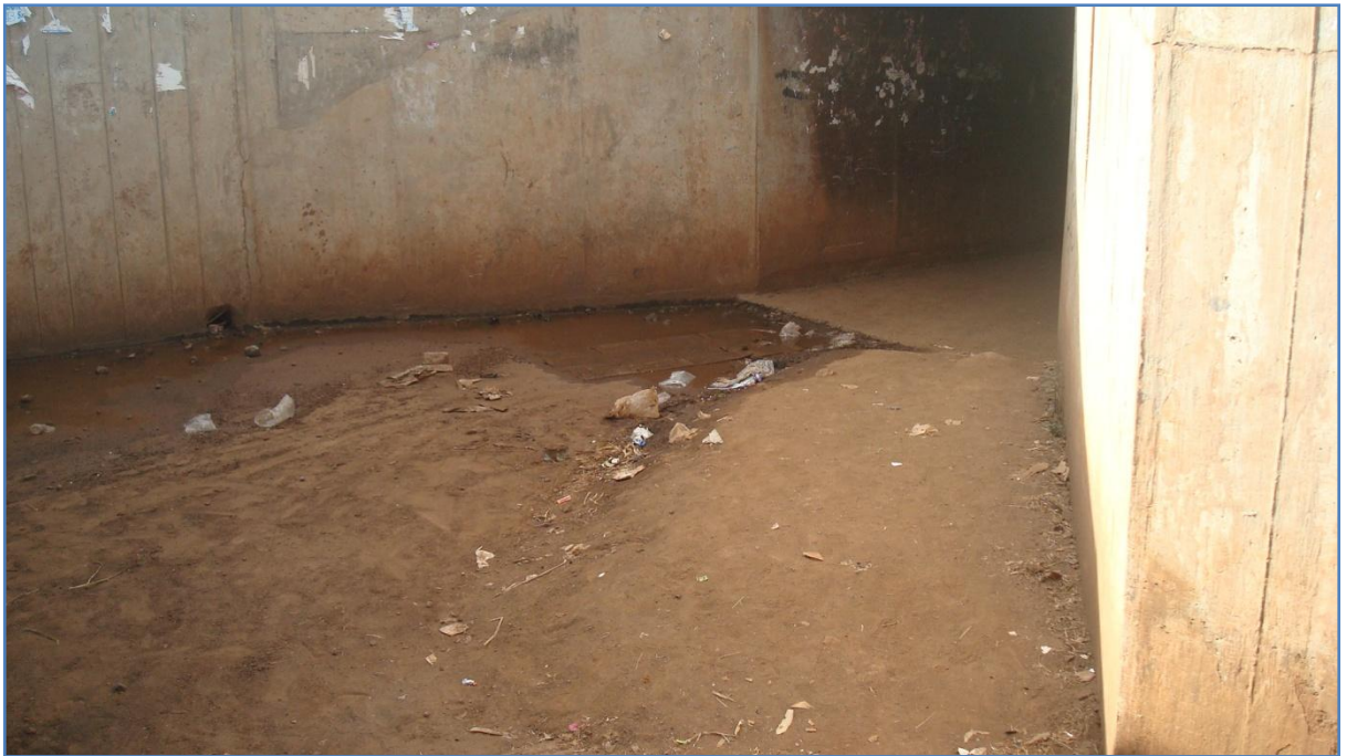
Picture 11: Mama Ngina Kenyatta Primary School Tunnel with debris at entrance
