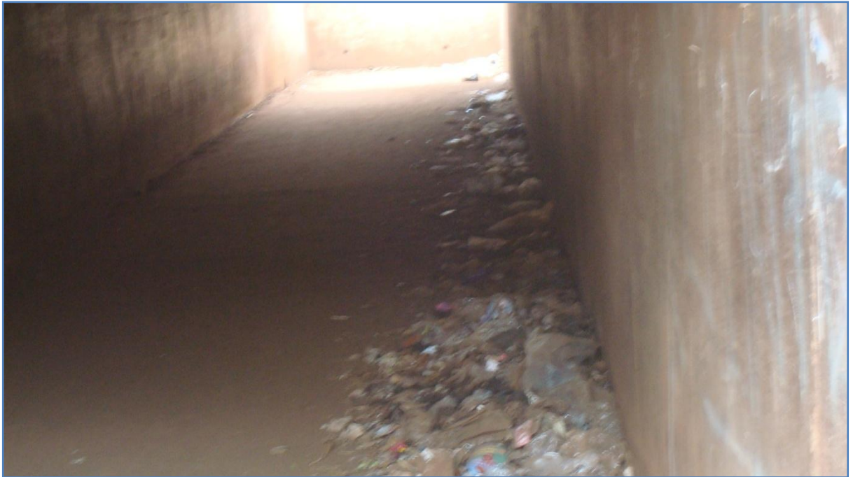
Picture 10: Mama Ngina Kenyatta Primary School Tunnel which is dark, unlit and with some rubbish
