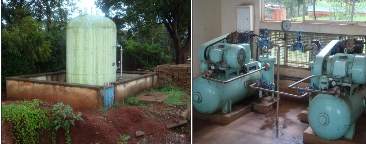
Fig 3-10: Surge Vessel and Air compressors. Source (NCWSC)
