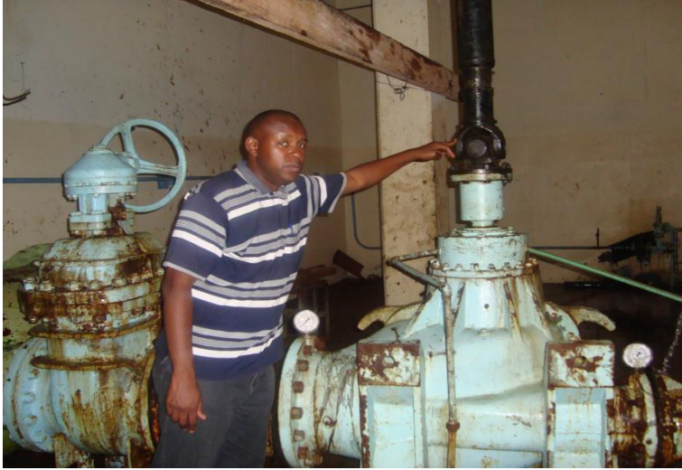
Fig 3-12: Propeller shaft universal joint on centrifugal pump input. (Author pointing at shaft universal joint) Source (NCWSC)
