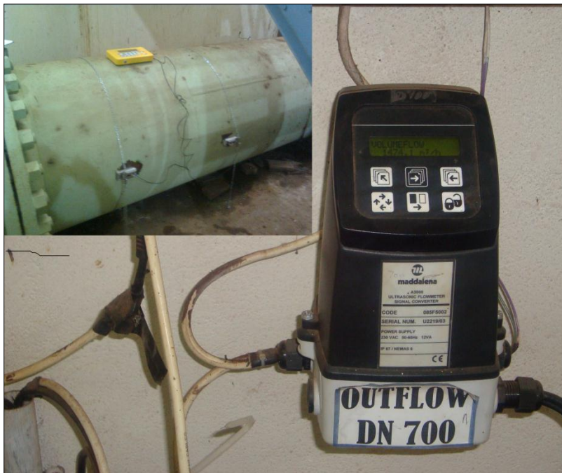
Fig 3-4: Pumping station flow meter (DN 700) and flow test set-up (Inset).Source (NCWSC & KEBS)
