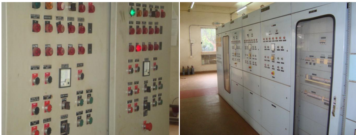
Fig 3-7: HV and LV switchboards. Source (NCWSC)
