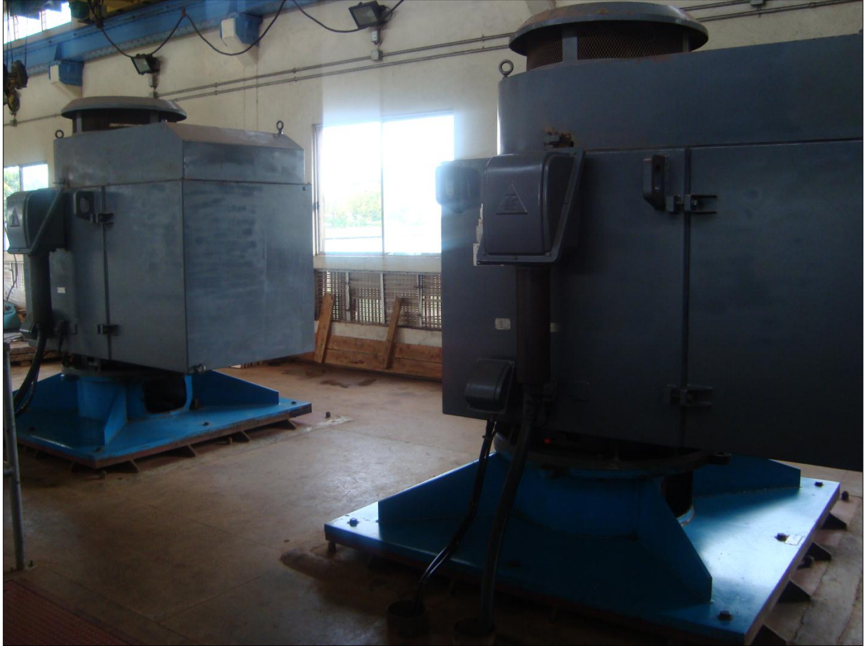
Fig 3-3: Vertical Electrical Motors for Pumps No. 3 and 4. Source (NCWSC)
