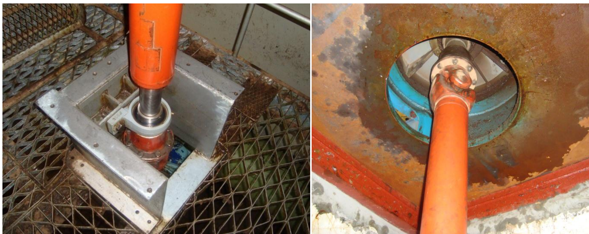
Fig 3-11: Propeller shaft on center bearing (left) and on motor output universal joint (right). Source (NCWSC)
