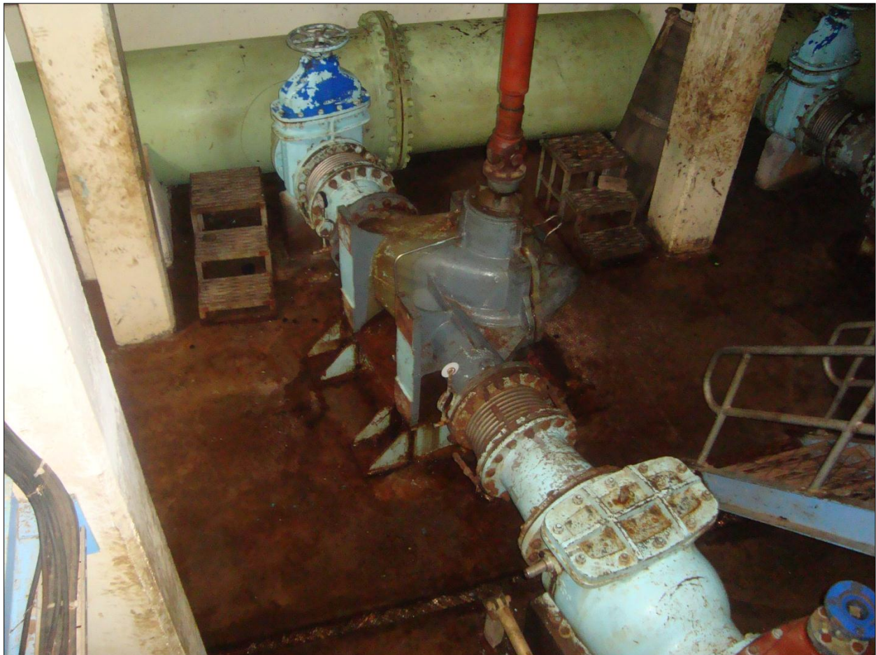
Fig 3-1: Pump No.4 Vertical Centrifugal pump as assembled with components. Source (NCWSC)
