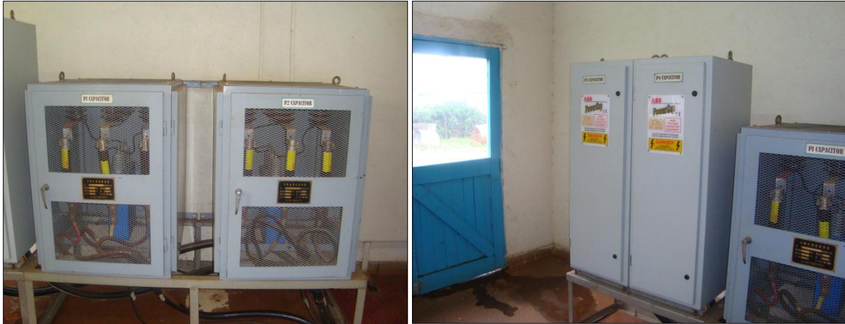
Fig 3-9: Capacitor banks for pumps No.1 and 2 (left) and No.3 and 4 (right). Source (NCWSC)
