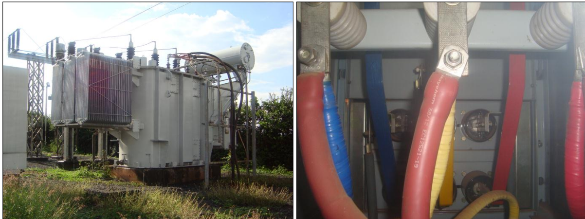
Fig 3-8: Sub-station 66 kV transformer and 3.3 kV bus bar terminating point. Source (NCWSC)
