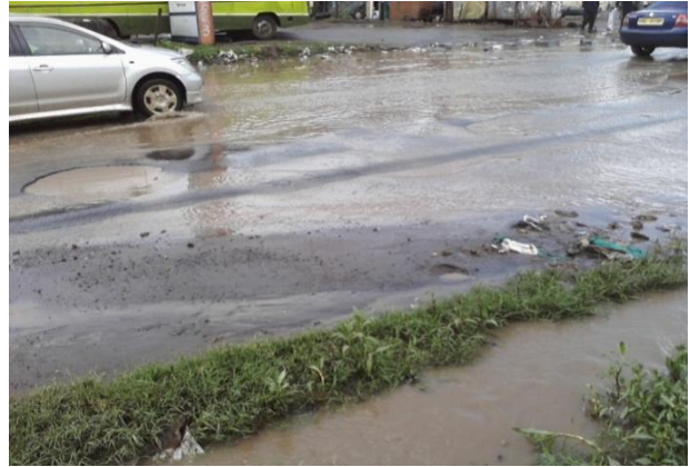
Fig 8 Appendix 1B A flooded road in Ongata Rongai town
