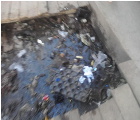
Fig 9 Appendix 1C An open septic tank behind Rongai market
