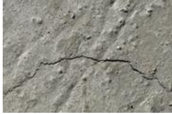
Figure 8: Plastic crack, Siaya, 2011.
