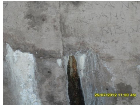
Figure 10: Efflorescence at a cold joint.
