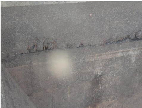
Figure 9: Poor compaction at a cold joint.
