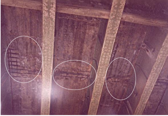
Figure 12: Rebar corrosion in a bridge soffit, road A109.
