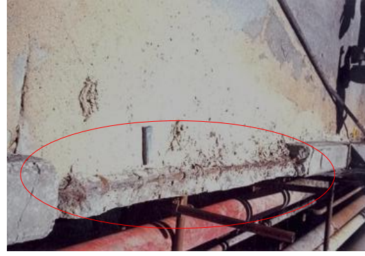
Figure 13: Rebar corrosion in a bridge within Mombasa port.
