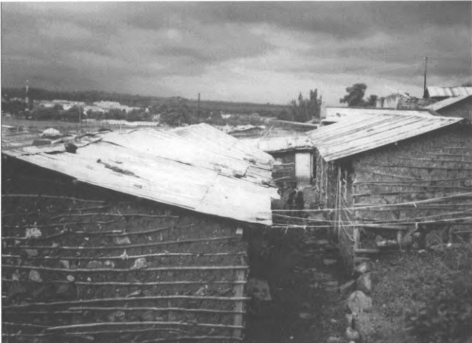
Plate 6-2: Poor Access to Housing Structures
