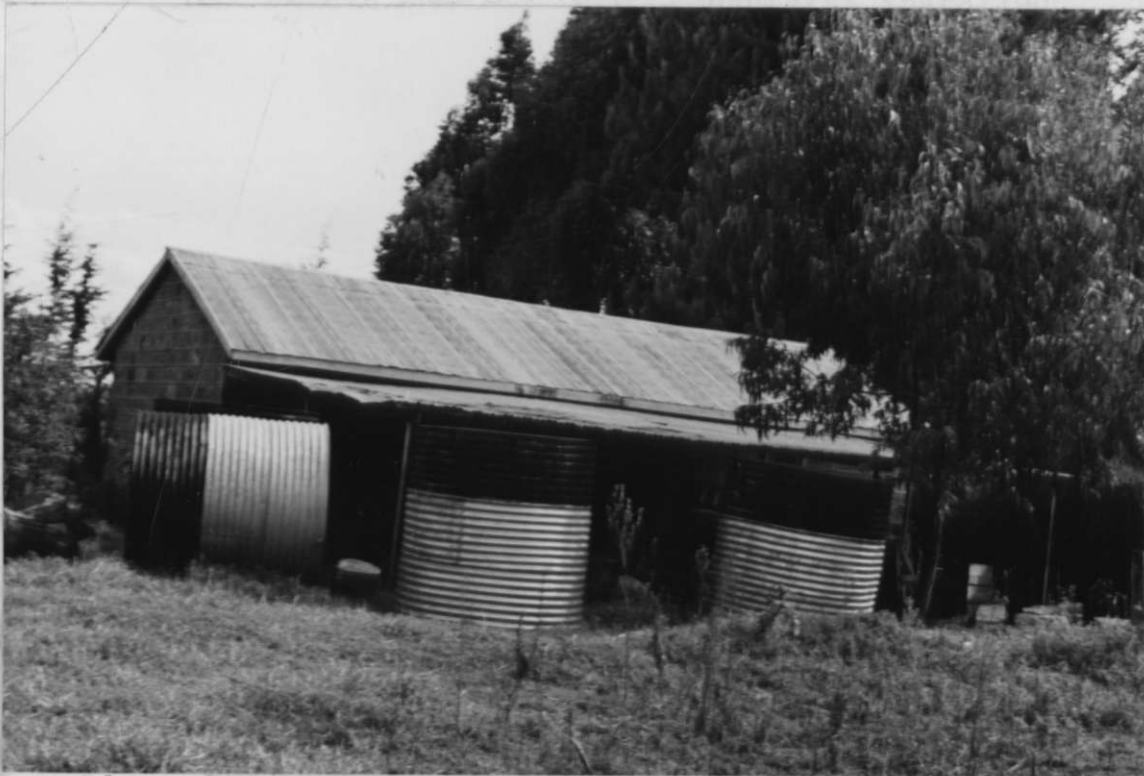
Plate 6: Roof catchment storage tanks made of corrugated iron sheets.
