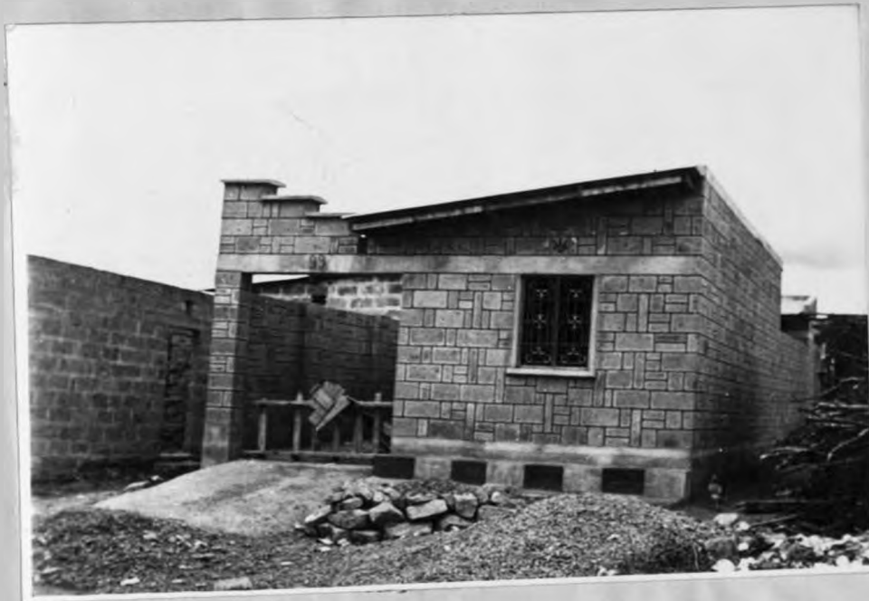
Plate No. 10 : Type B plot suspected sold - note the expensive building materials used e.g. roofing tiles. Estimated cost of construction Shs. 145,000.
