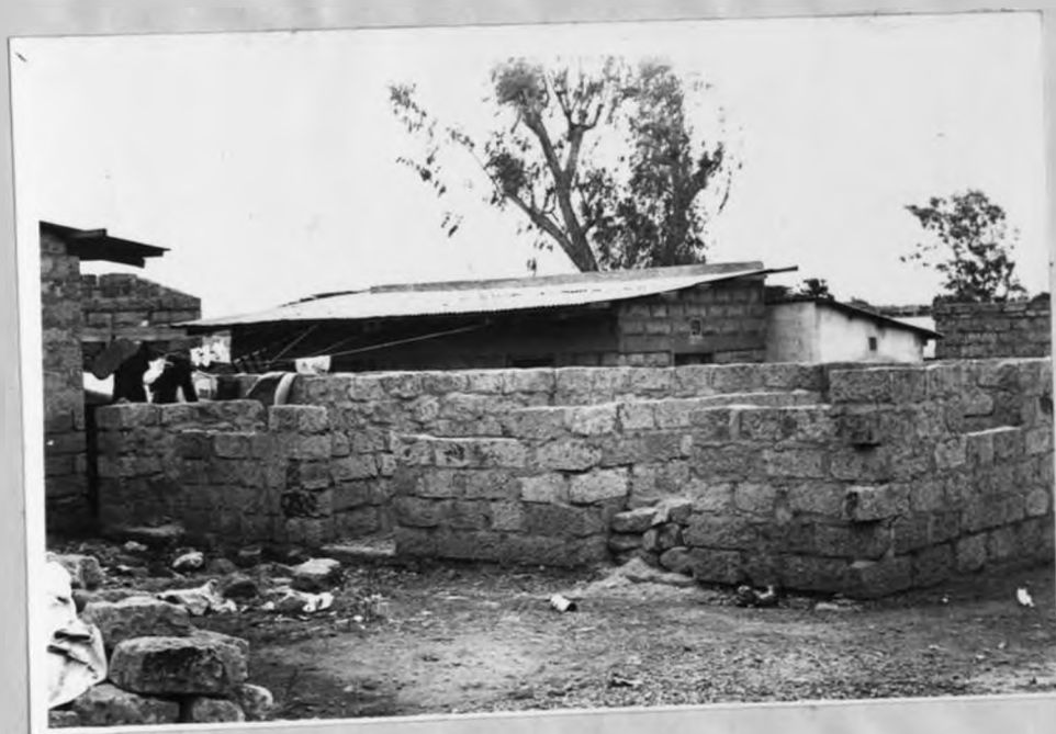
Plate No.8: A type A plot being erected in whole after sale.
