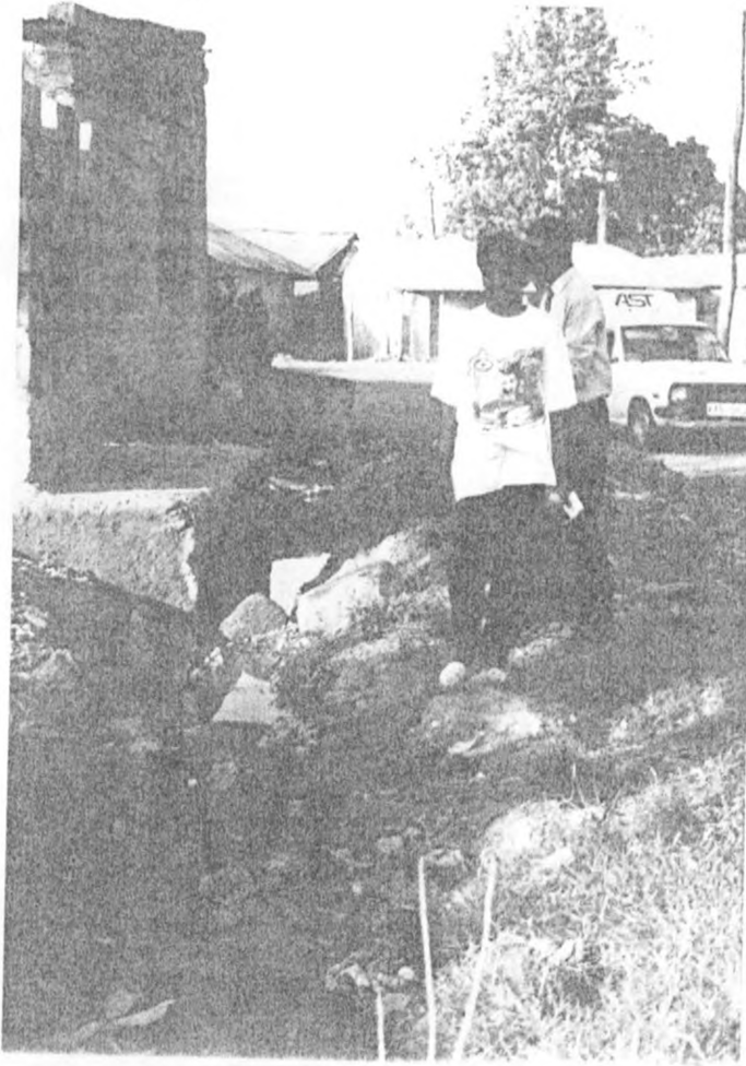
Plate 13: Poorly maintained storm water drainage channel in part A
