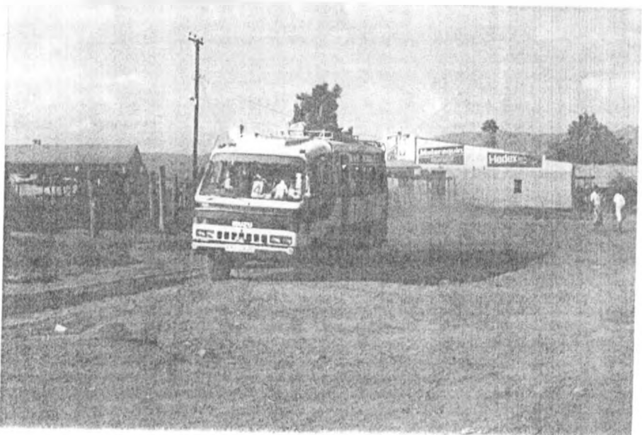
Plate 12 The formally well constructed tarmac roads are under serious conditions of disrepair (part A)
