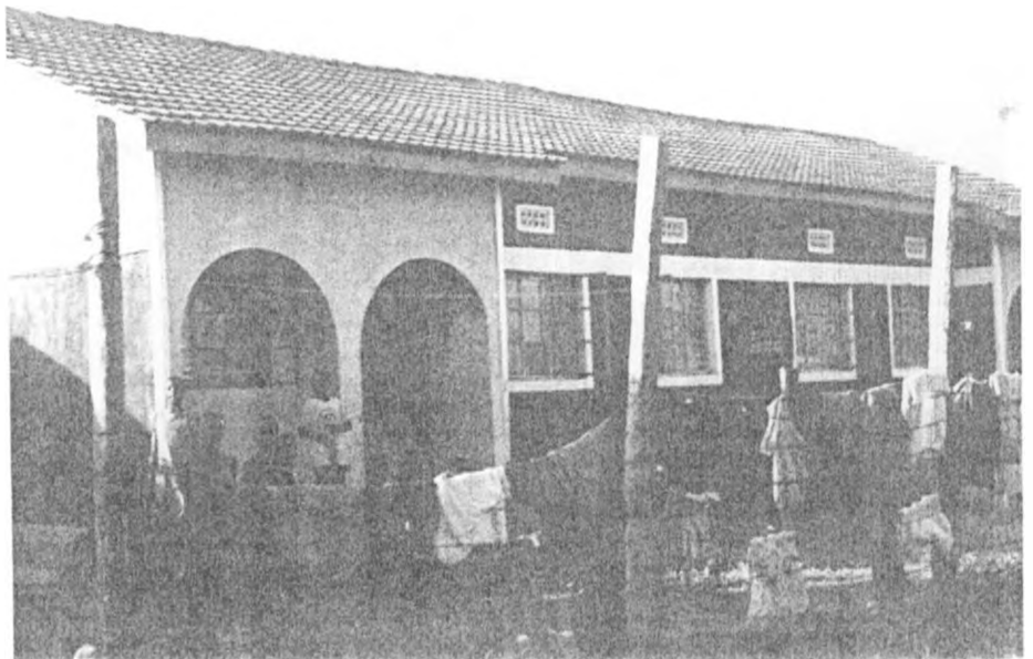
Plate 6 A block of semi-detached bungalows exhibiting high structural soundness in part B
