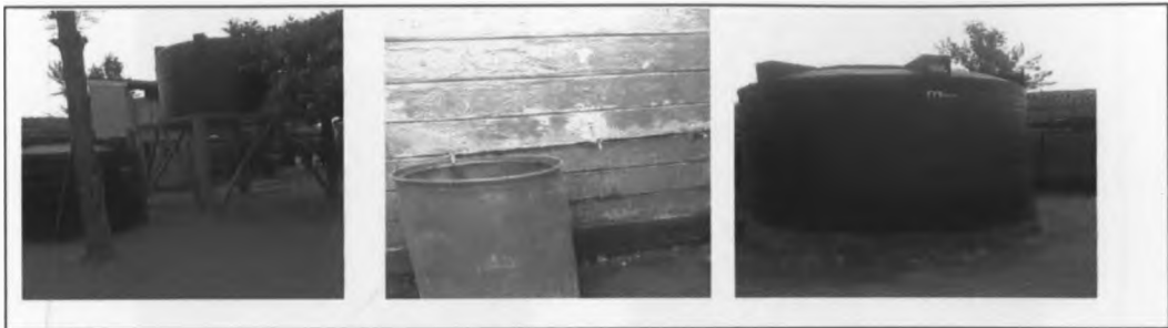
Water tanks and taps for hand-washing
