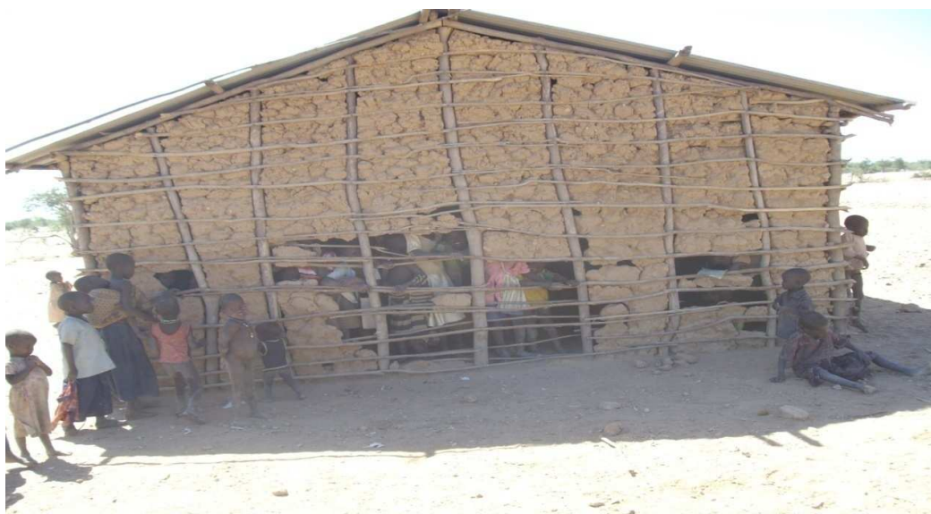
Plate 20: Dilapidated and crowded classroom
